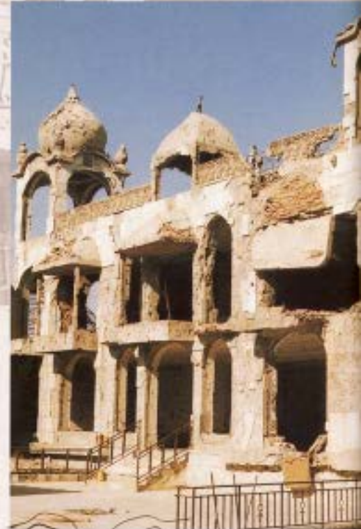
....and seen damaged, above.
