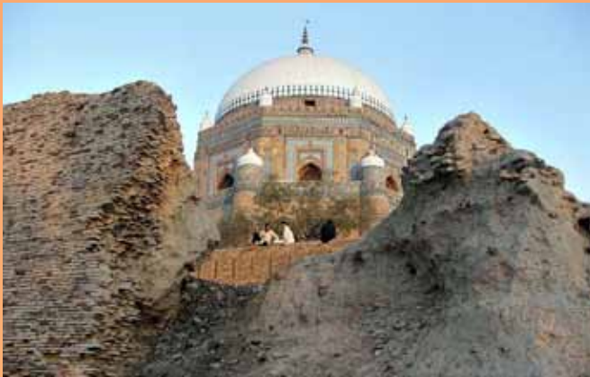
A dilapidated outer boundary wall of the Multan Fort
